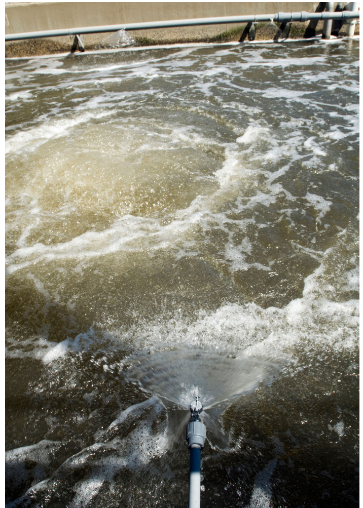
Sewage treatment - aeration
